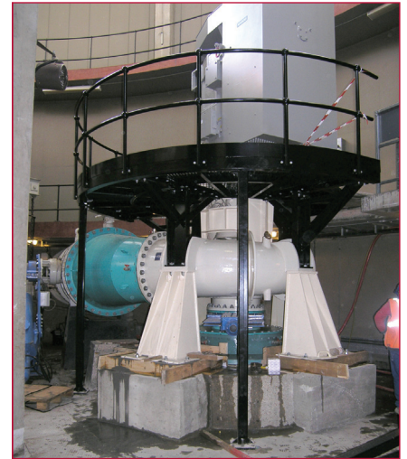
The Bedford Pumps DV.90.23.10 Volute pump has been installed at Thames Water's Datchet Pumping Station (above). Driven by a 6.6kV variable speed motor, this pump has a rated flow of 50 to 225 million litres a day. The assembly is fitted with four accelerometers and seven temperature sensors, all feeding into a Monitran MTN/6000 monitoring unit.
