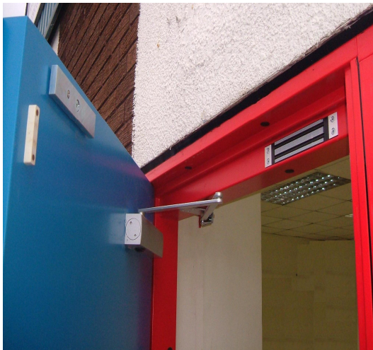
Recessed Head Magnet for remote or keypad Access. Vertical magnets x 2no available for Added strength. Door core should be upgraded To solid timber core to suit this application
